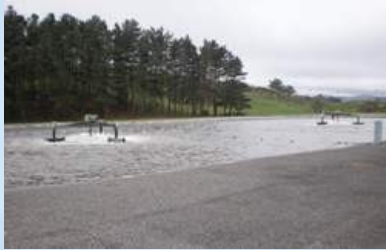
Figure 7 - Vertical propeller aerator
