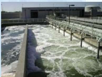
Figure 5 - Bottom air Diffusion in operation
